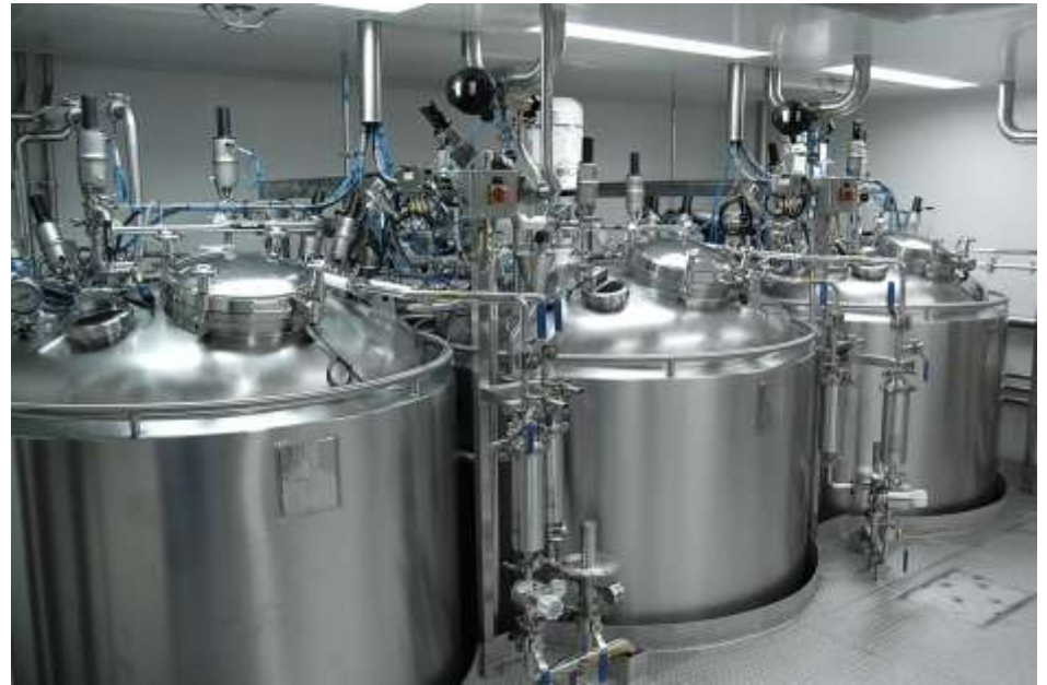
Cuve de Process
